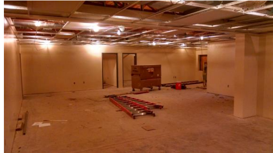
Federal Programs Offices – Drywall Complete, Painting, Ceiling Grid Installation, HVAC Above Ceiling Duct Installation, and Lighting Installation
